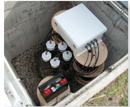
Piezometers and Extensometers
